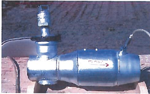
Chemigation check valve. The 2 bolts on top show the location of the spring operated flapper. Note the 4 inch inspection port with the air release valve on top and the injection port downstream from the flapper location.
