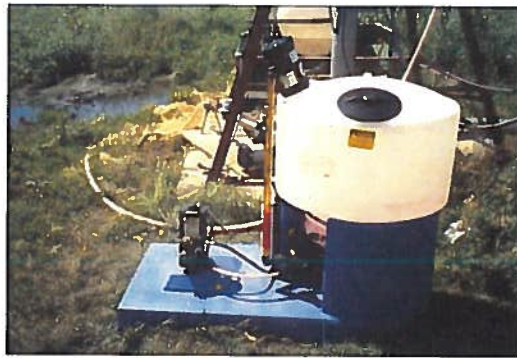
Typical modular chemical injection equipment. Note the calibration tube on side of tank and the mixing motor on top of tank.
