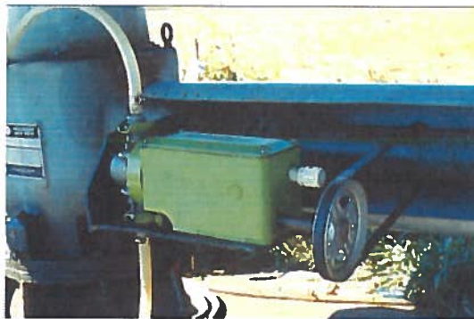
Mechanical interlock shuts off the chemical injection pump when the water pump stops. Note the drive belt around the drive shaft of the water pump.
