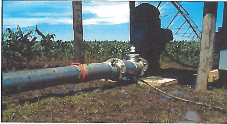
Chemigation check valve next to the well. Note the rubber hose connected to the low pressure drain directs leaking water away from the well.
