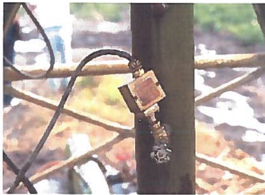
Pressure sensor on the riser pipe of a center pivot. If a low pressure situation occurs, the well pump, chemigation pump and pivot should shut down.
